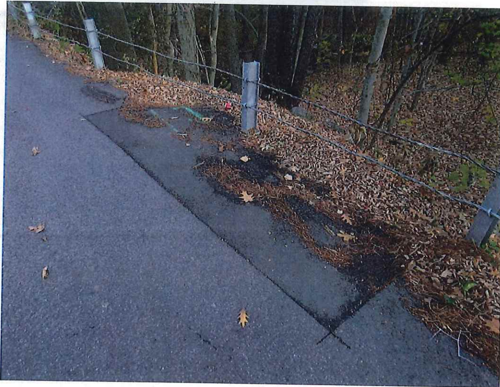
Photo 3: Bituminous patch to the Northbound lane of the South approach.
