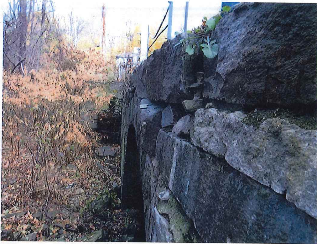
Photo 7: Displaced stones on the West spandrel wall.
