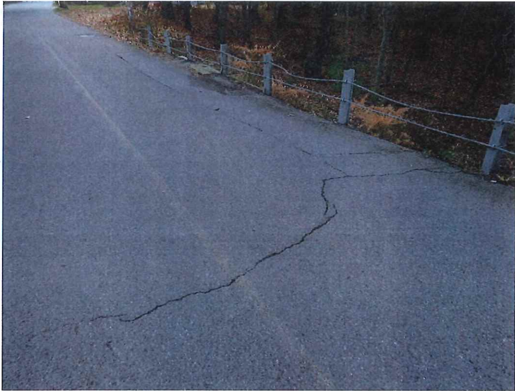
Photo 1: Transverse crack to the wearing surface near midspan.
