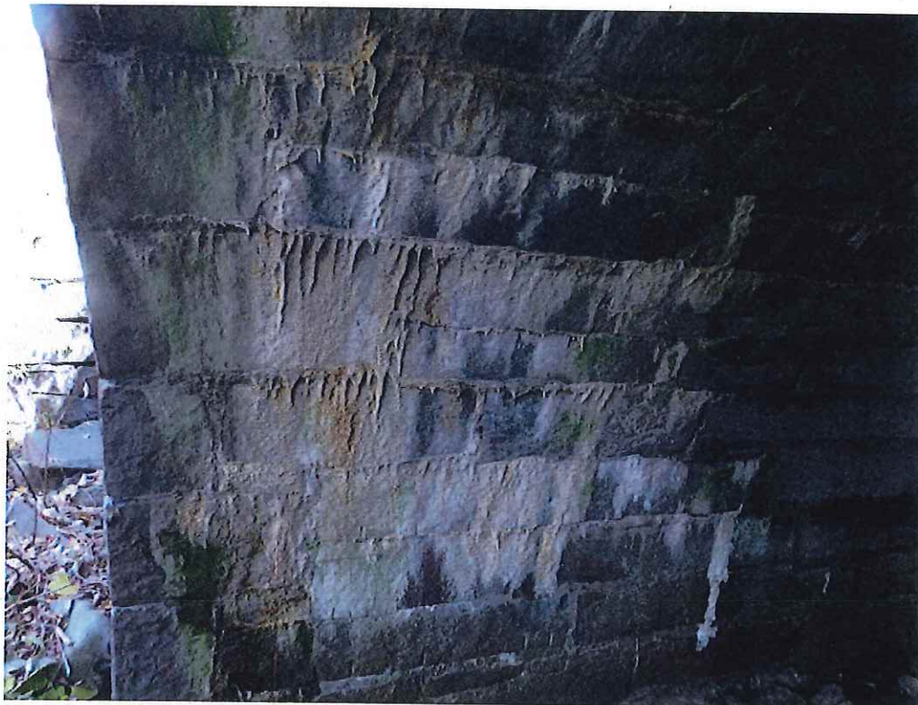
Photo 12: Heavy efflorescence to the Northwest corner of the arch.
