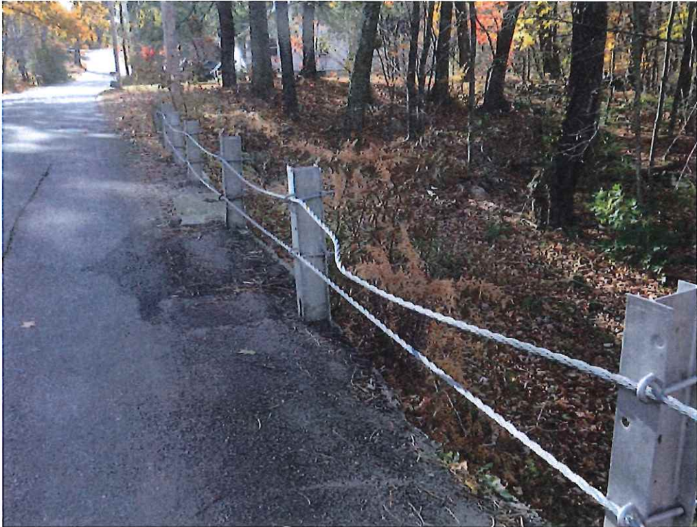
Photo 2: Loose top West cable.
