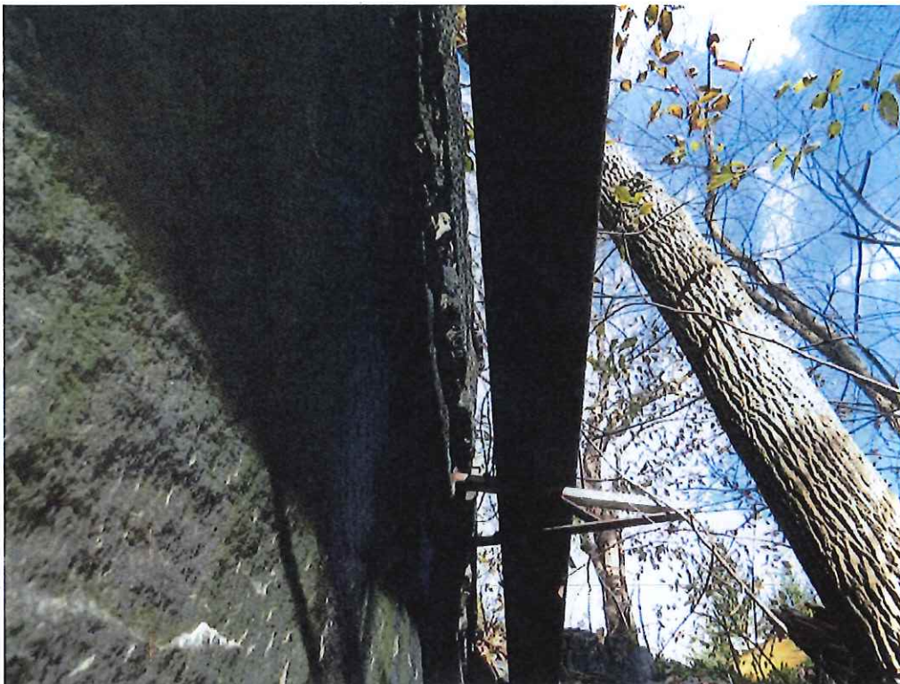
Photo 10: Displaced top stones on the North half of the East spandrel wall.
