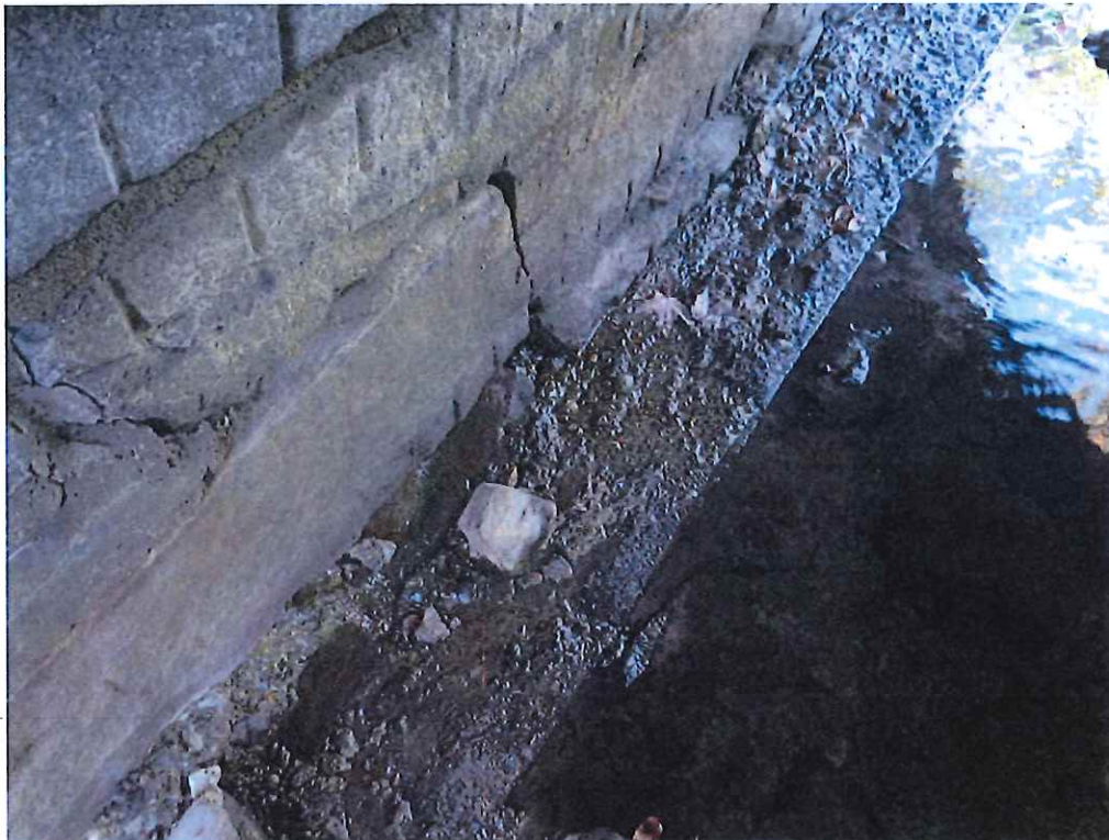
Photo 14: Typical condition of the North footing and leakage through the North breastwall.
