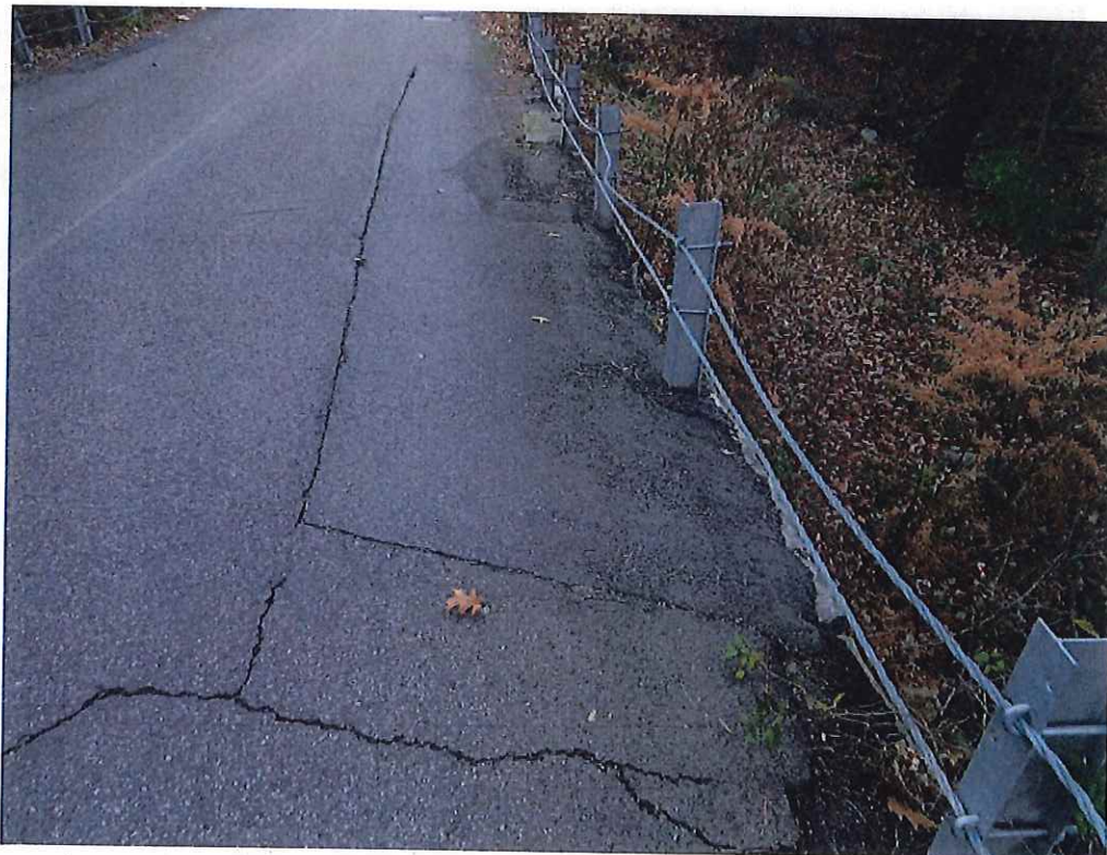
Photo 4: Bituminous patch to the Southbound lane of the South approach and wearing surface.
