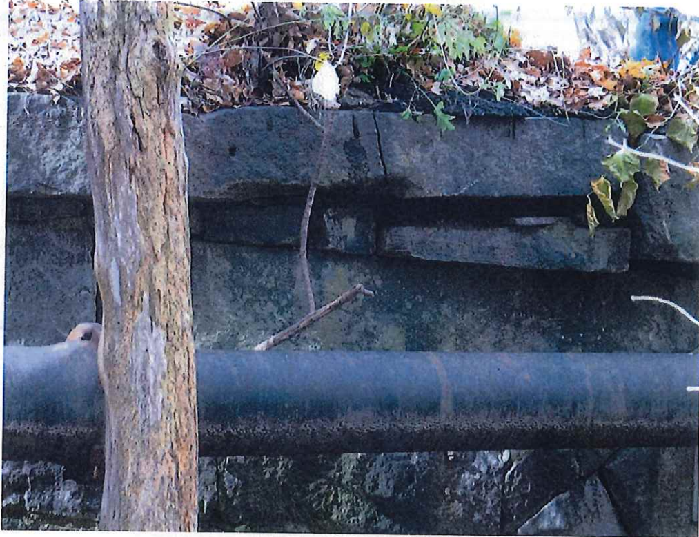
Photo 11: Cracked stone on the top of the East spandrel wall near the South end of the arch.
