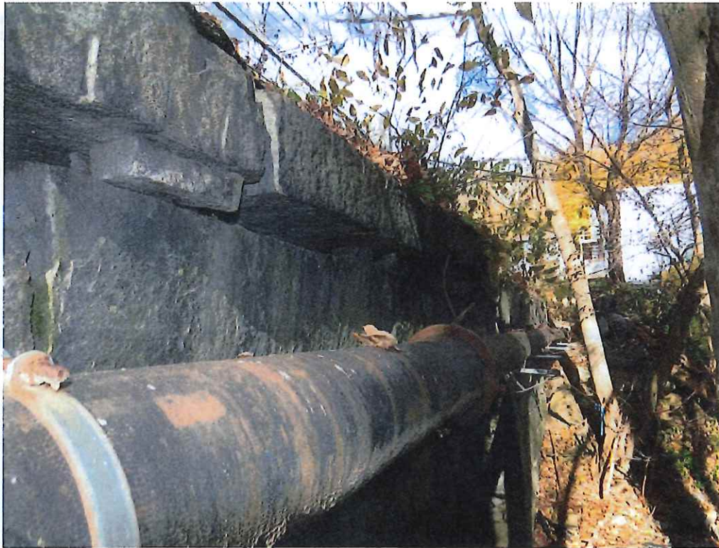
Photo 9: Displaced top stones on the South half of the East spandrel wall (view from below).
