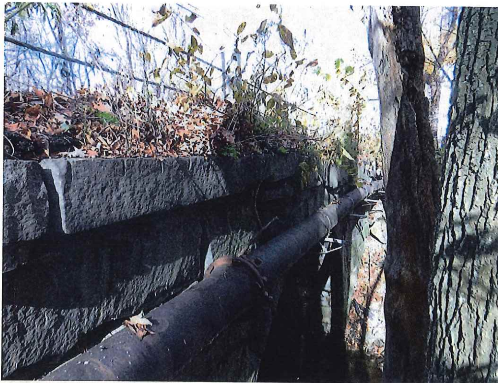
Photo 8: Displaced top stones on the South half of the East spandrel wall.
