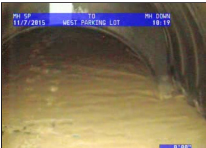
SEPARATOR ROW: Separator Row prior to cleaning
