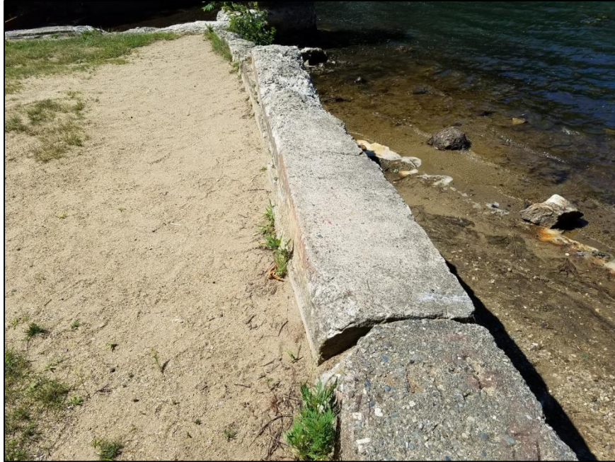
Photo 17: Leaning upstream wall
