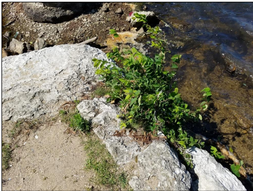
Photo 20: Woody vegetation growing through upstream wall
