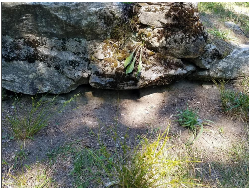
Photo 26: Burrows observed in downstream left stone retaining wall
