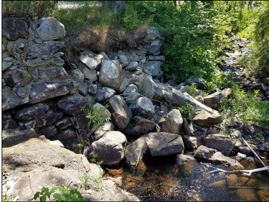
Photo 21: Collapsed downstream training wall
