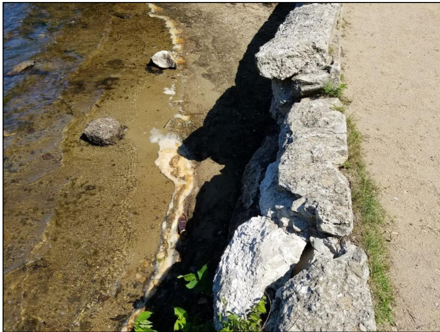
Photo 18: Deteriorating upstream wall
