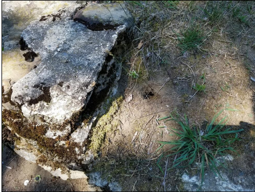
Photo 25: Burrows observed in downstream left stone retaining wall
