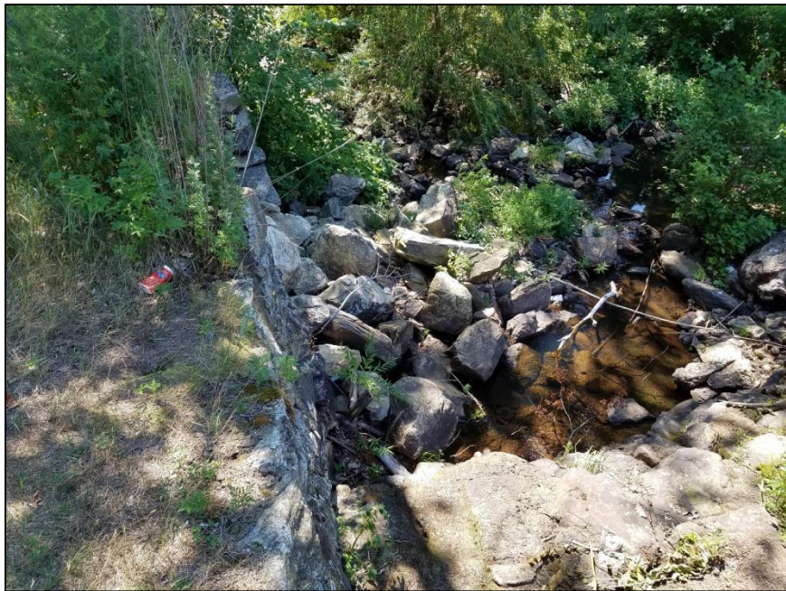
Photo 22: Collapsed downstream training wall
