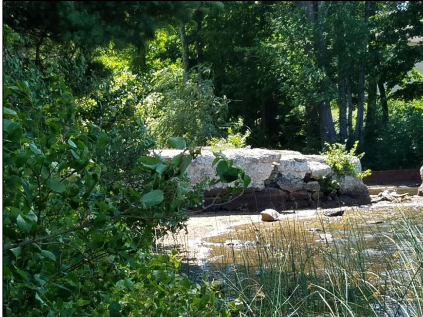
Photo 19: Deteriorating upstream wall
