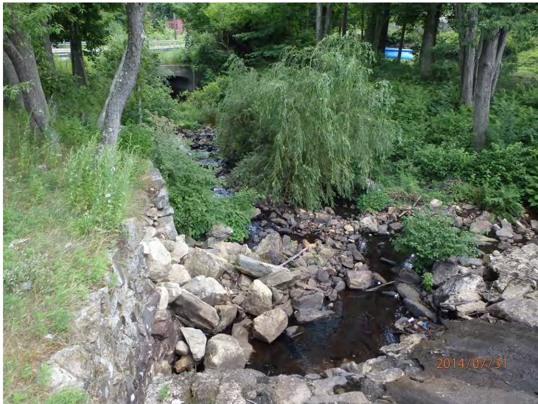
Photo 15: Areas of specific deficiencies-failing downstream channel wall
