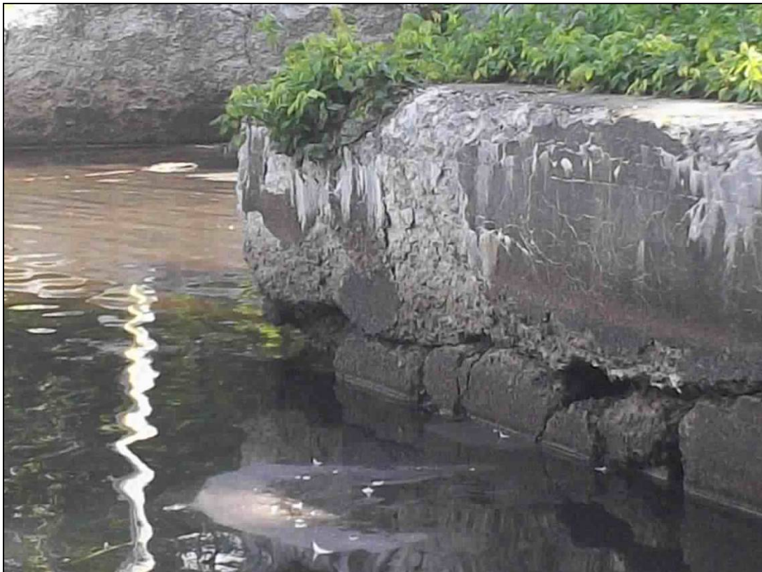
Photo 23: Areas of specific deficiencies-undermined cracked wall
