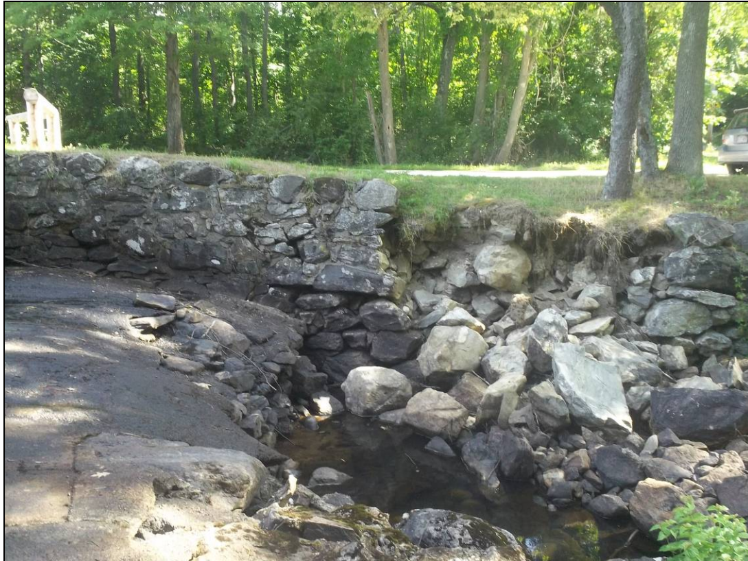
Photo 22: Areas of specific deficiencies-collapsed masonry wall
