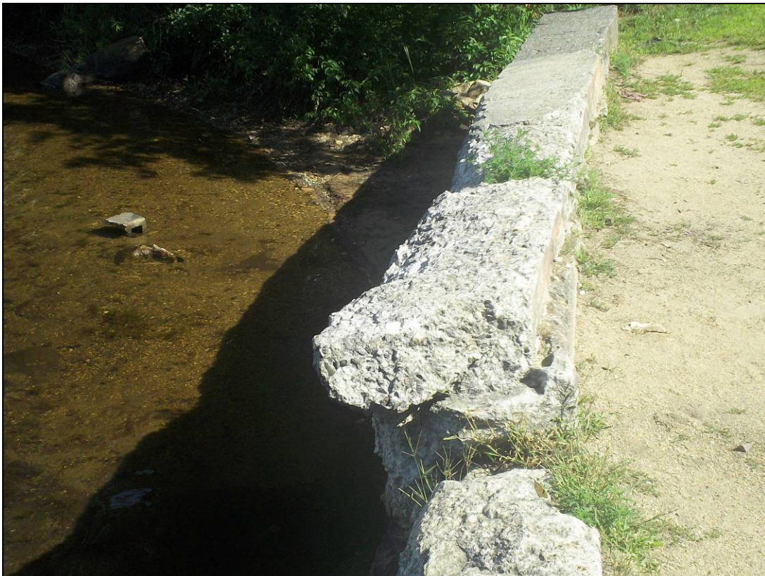
Photo 21: Areas of specific deficiencies-deteriorating concrete, leaning wall
