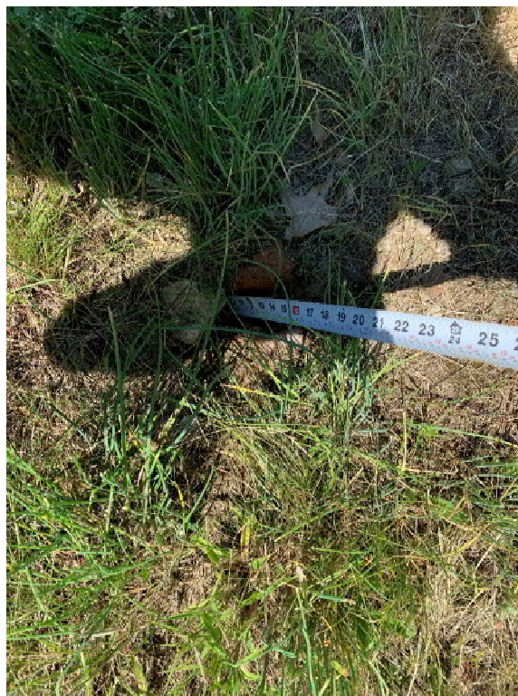
Photo 30: Animal burrow #2 on the downstream slope (area of specific deficiencies)
