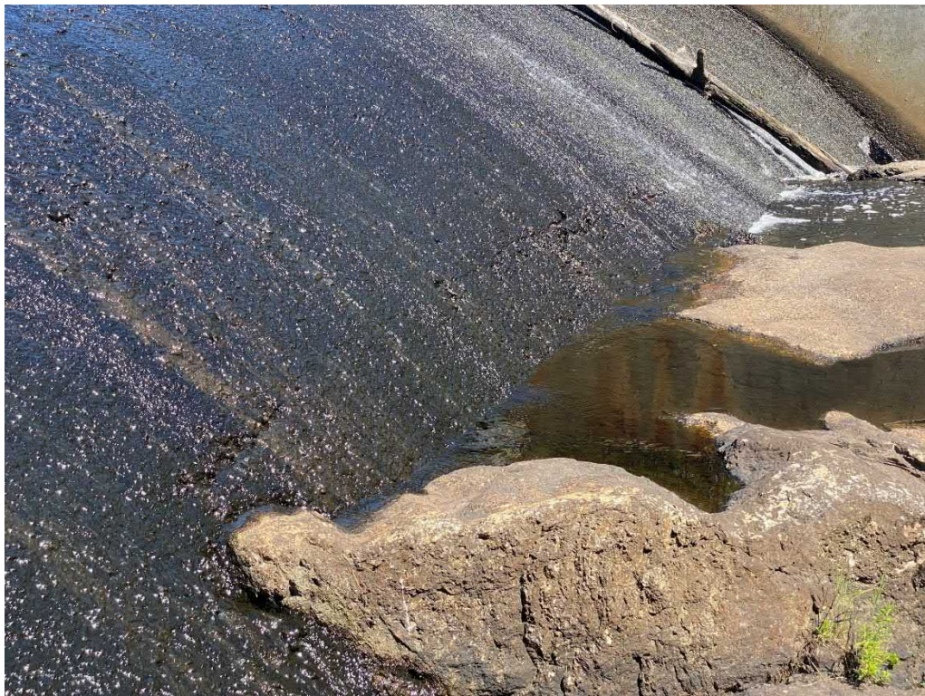
Photo 24: Concrete erosion in ogee weir face
