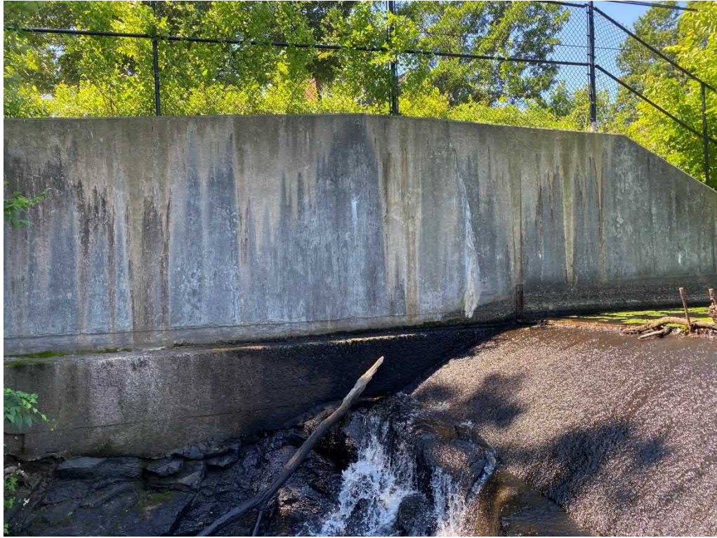
Photo 23: Cracks in right training wall
