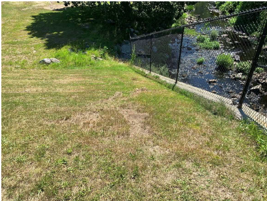
Photo 28: Minor erosion and bare spots on downstream slope
