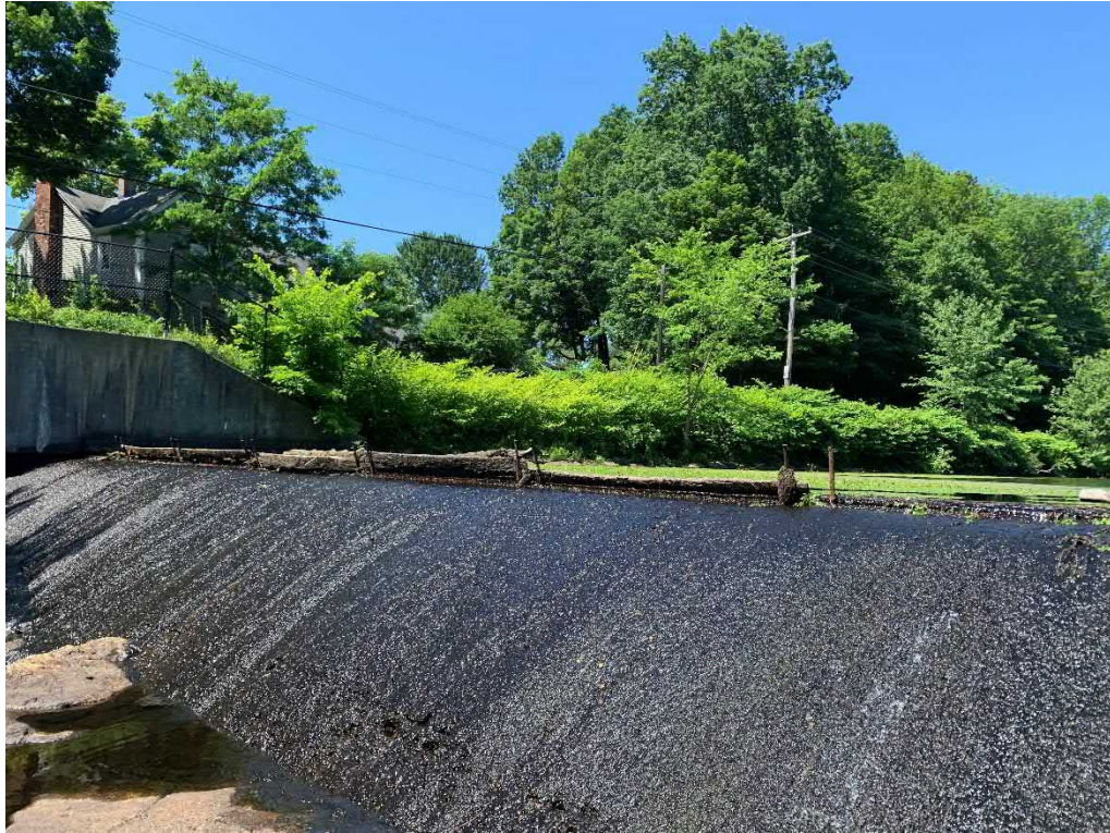
Photo 27: Overview of spillway flashboards (note missing boards)
