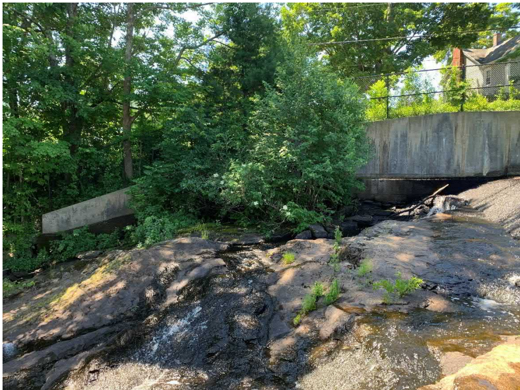
Photo 22: Vegetation growing in spillway channel near right abutment
