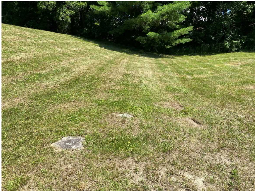
Photo 26: Previous sloughed area on downstream embankment – now vegetated and stable
