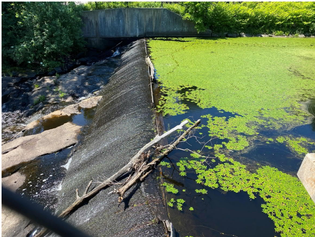
Photo 12: Overview of weir – note debris, failing flashboards
