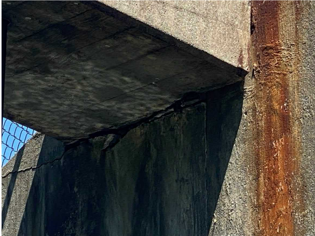
Photo 25: Cracked concrete in cantilevered gate operator pedestal and training wall
