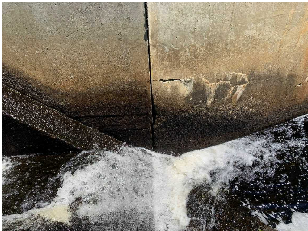
Photo 20: Crack and deteriorating joint left training wall
