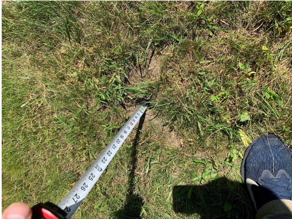
Photo 29: Animal burrow #1 on the downstream slope (area of specific deficiencies)
