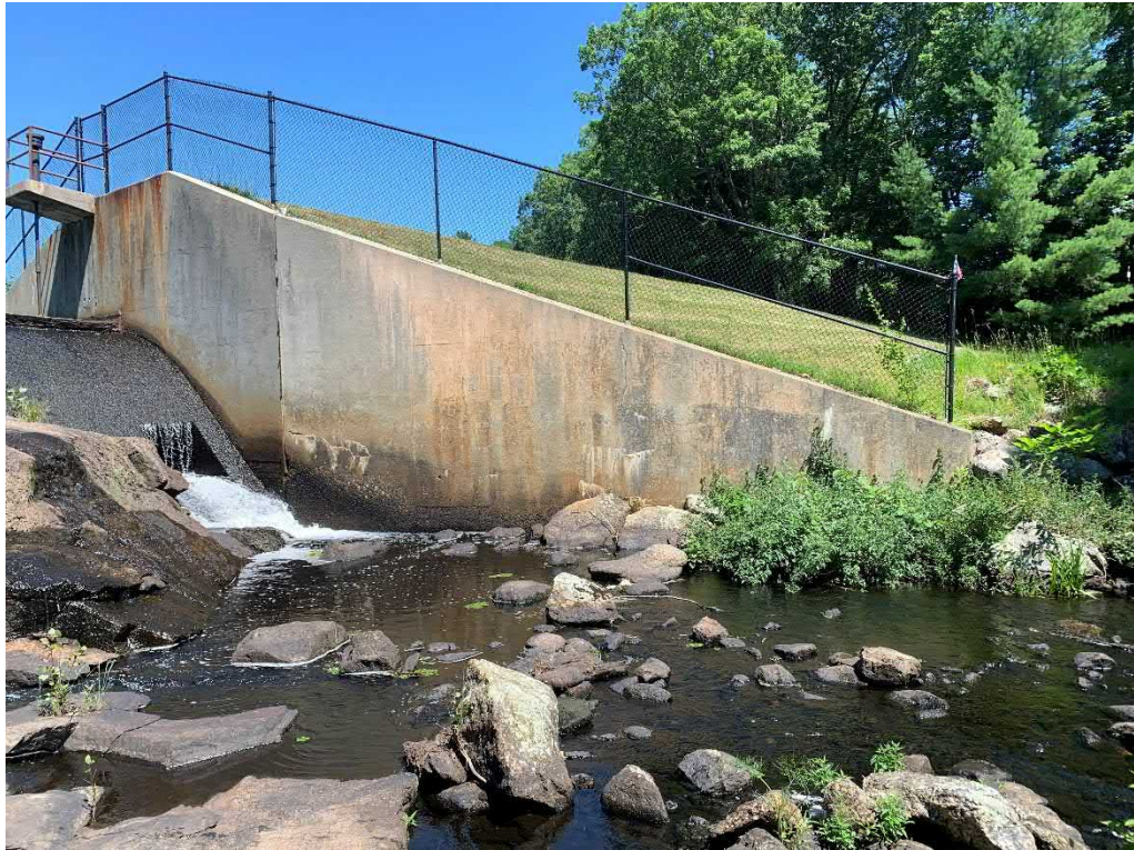
Photo 21: Cracks in left training wall
