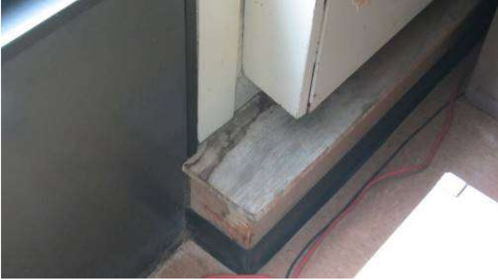
Water-damaged wood beneath radiator valves
