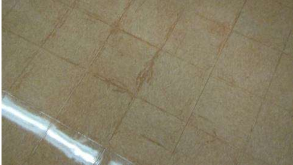
Staining of floor tile edges can be a sign of repeated condensation exposure
