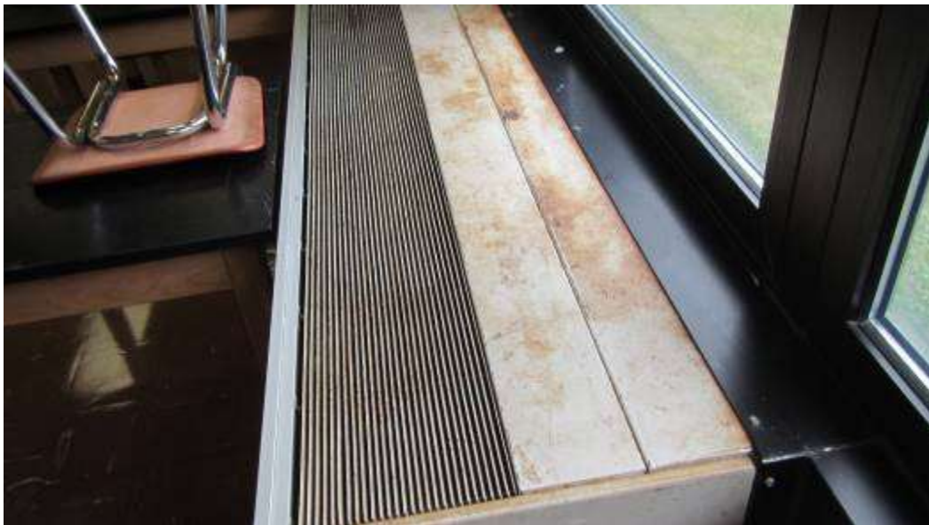
Univalent corrosion, exterior
