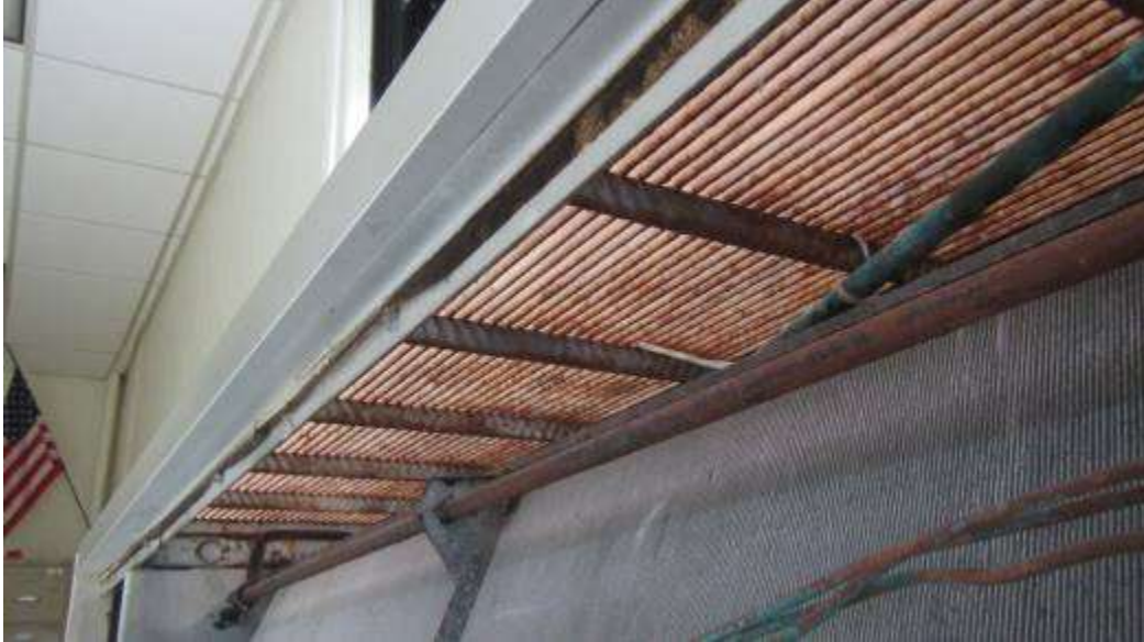
Univalent corrosion, interior
