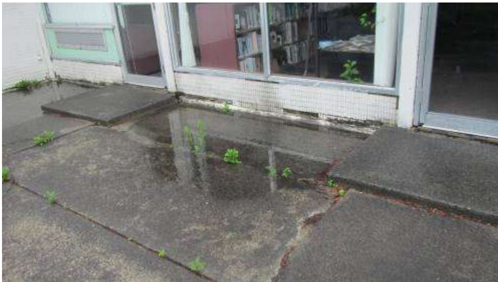
Water pooling against library exterior courtyard wall
