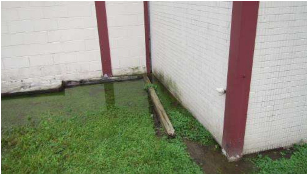
Furrow-like depression of exposed dirt adjacent to the building slab, note pooled water
