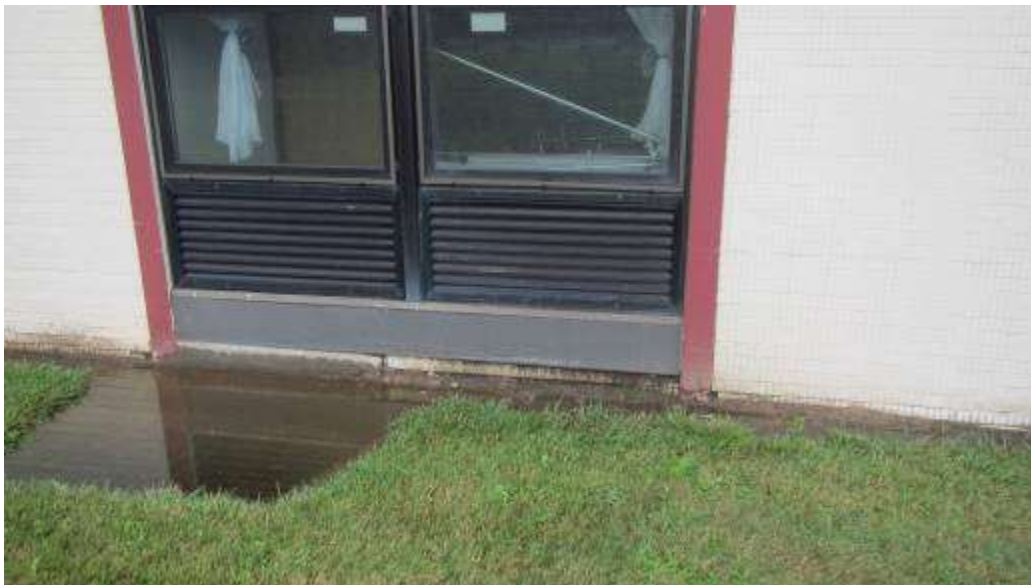
Univent fresh air intake, note pooling water
