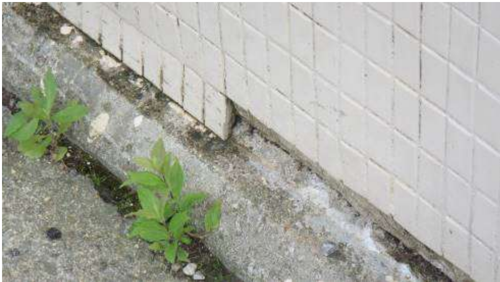
Damage at the exterior wall/slab junction; note no flashing at this joint
