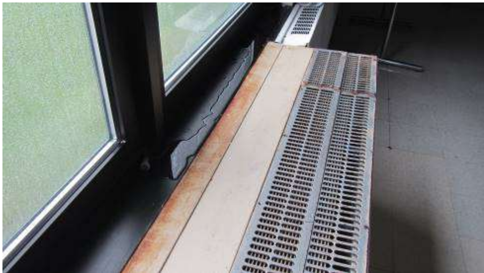
Rainwater on windowsill
