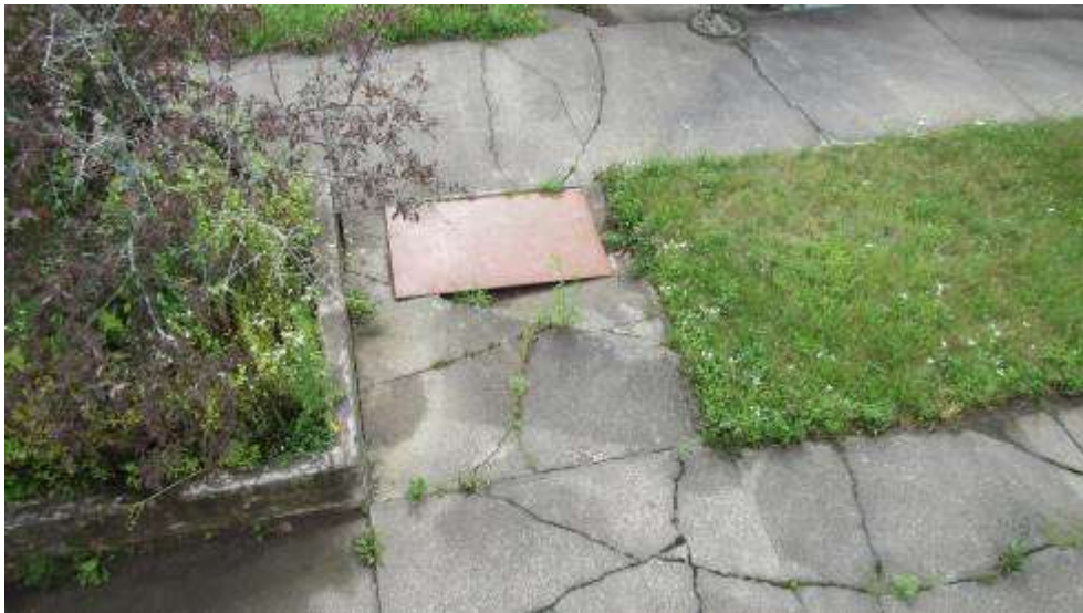
Metal plate covering sink hole
